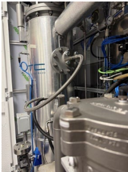
1. Hydrogen Conditioning Loop
